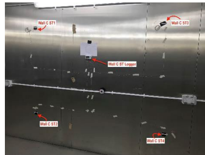
Wall surface temperature sensors
